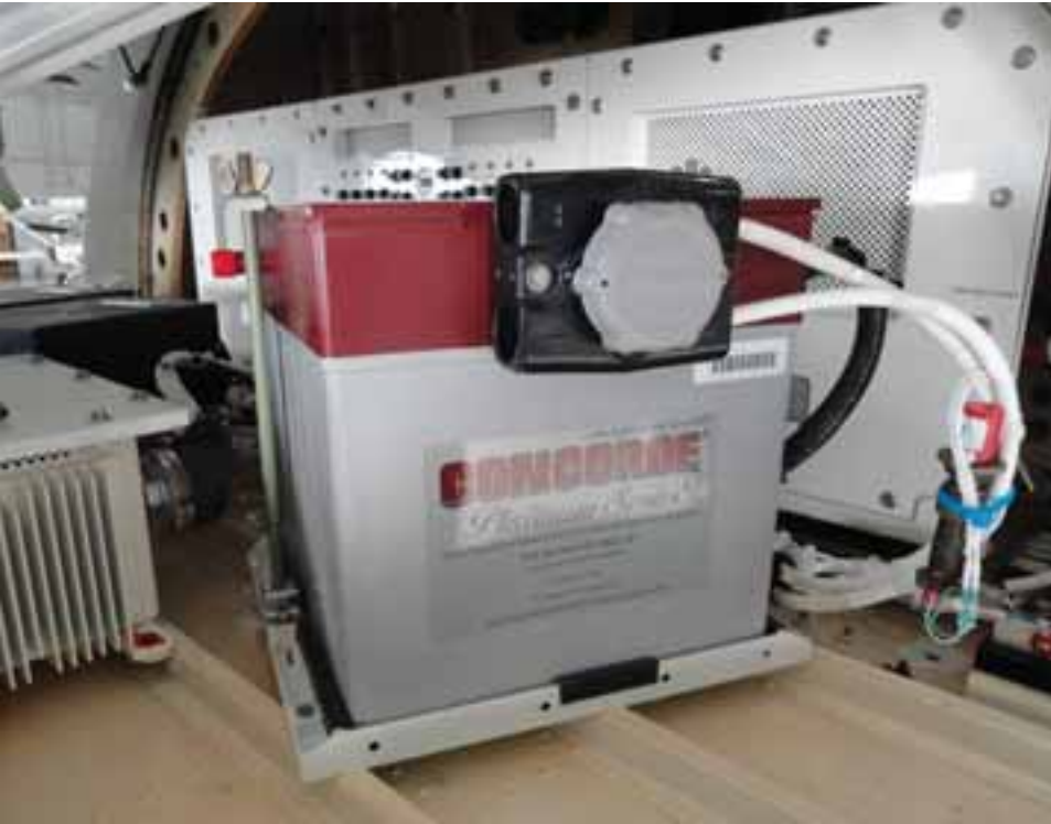
Concorde RG-380E/44 battery installed in a DHC-8 aircraft.
