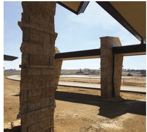
Crews finish up the access road to the new terminal. Joe Petrie/Airport Business
