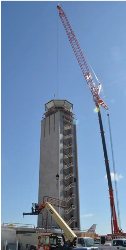
The south tower's cab glass is hoisted into position using a crane.
