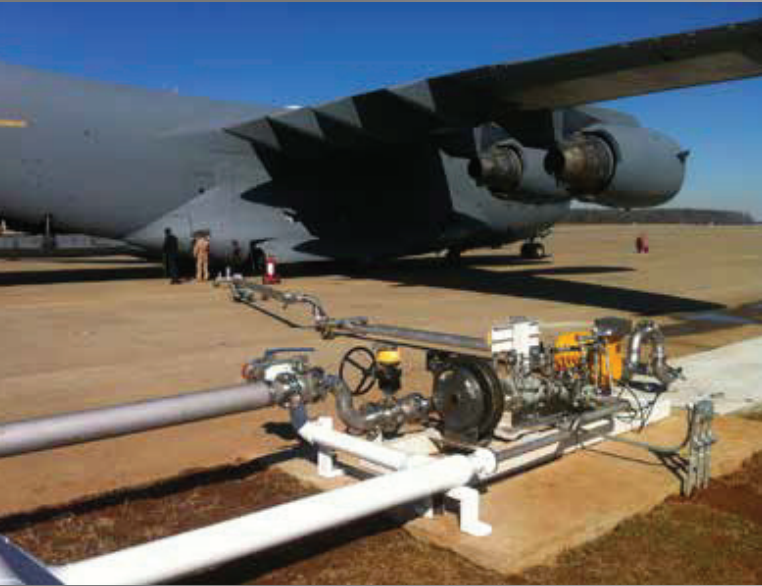
Pantograph Fueling Systems
