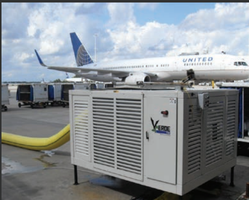
Verde 60 Ton PCA system at Orlando International Airport
