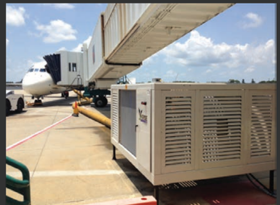
Verde 60 Ton PCA system at Sarasota International Airport
