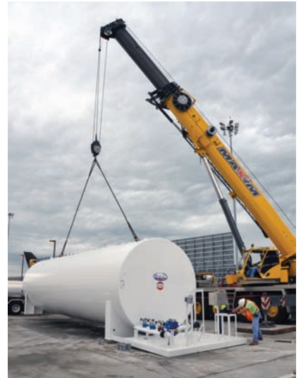
UPS installed two biodiesel tanks at Worldport last March to provide customized fuel for about 200 diesel-powered GSE.
