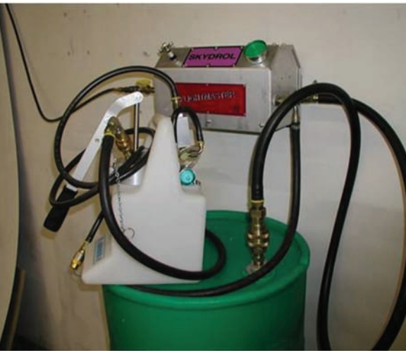
A complete closed-containment system: wall-mounted pump; bung kit and dispenser.
