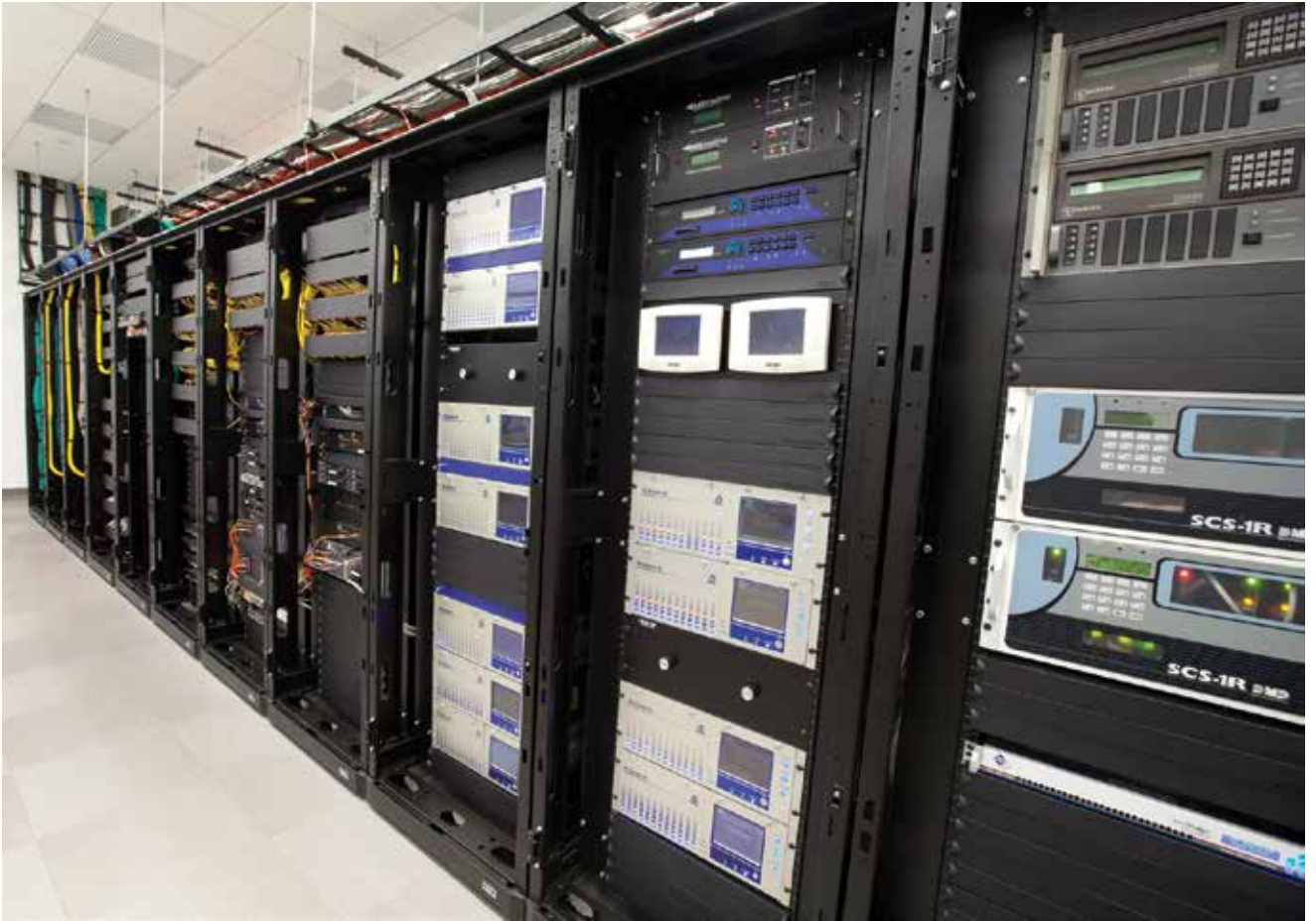
Affiliated Monitoring provides robust managed access services to its dealers, who retain their identity with the customers.
