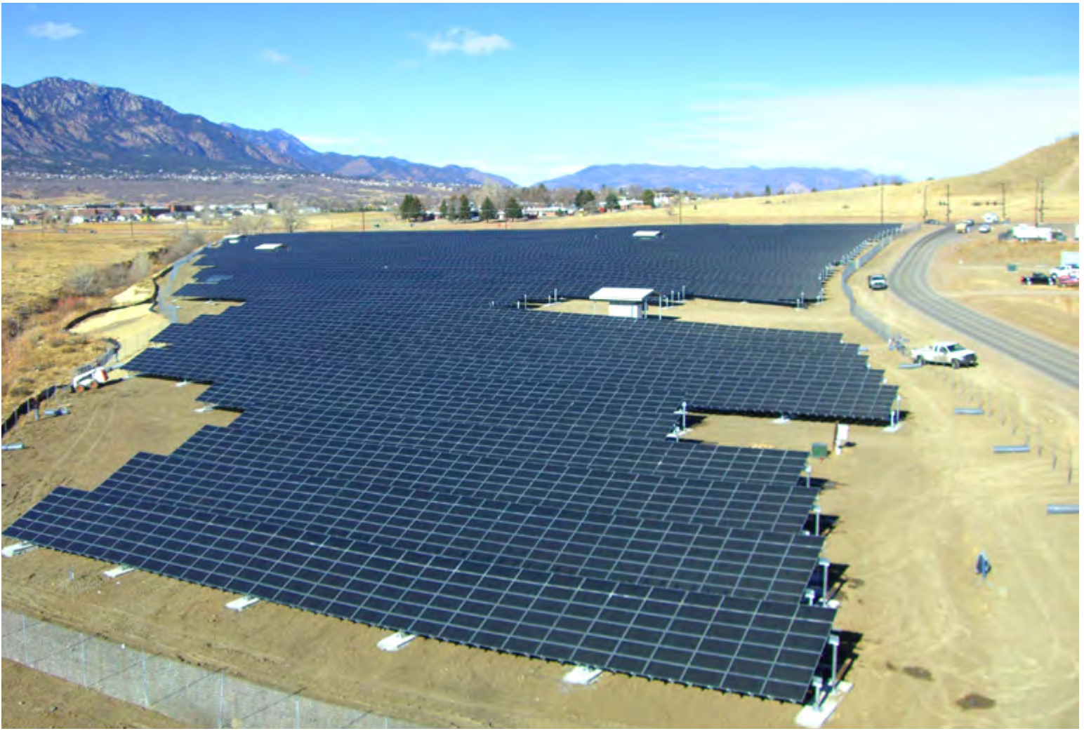
Solar photovoltaics at Fort Carson, CO
