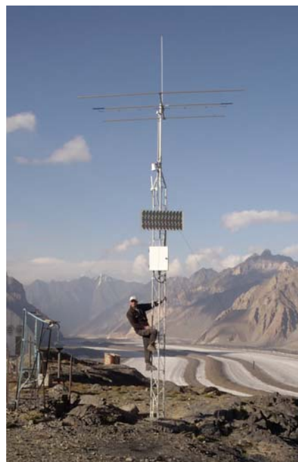
SunWize® Power Ready System in Tajikistan.
