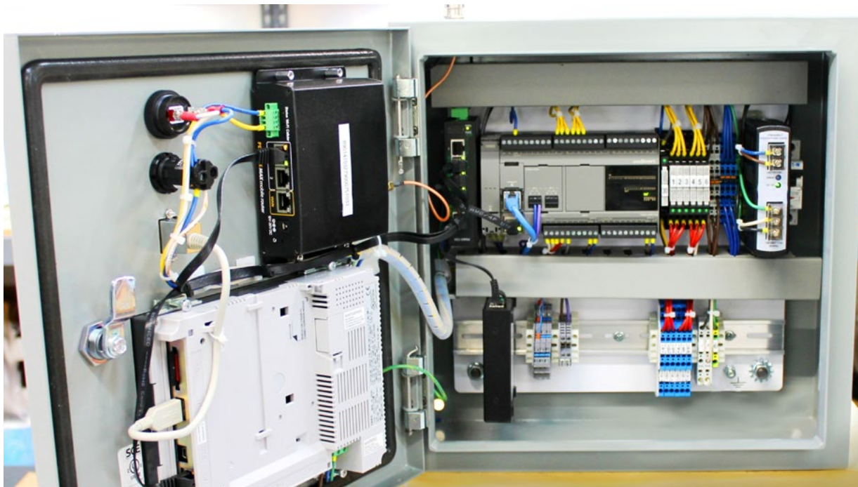
Figure 3. The entire control system including the PLC, the HMI and other ancillary components is housed in a small enclosure, saving money and space.
