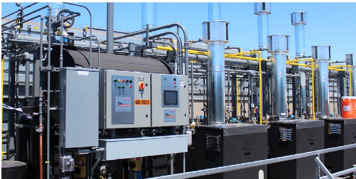
Figure 1: Modular systems from Parker Boiler provide improved performance as compared to one larger boiler, as with these four smaller boilers.
