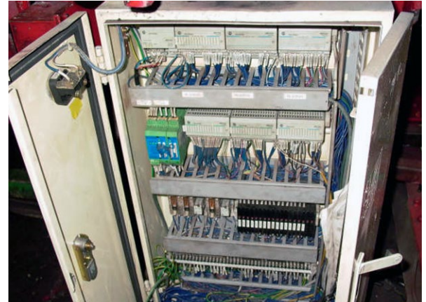
Figure 2: Cabinet mounted I/O example
