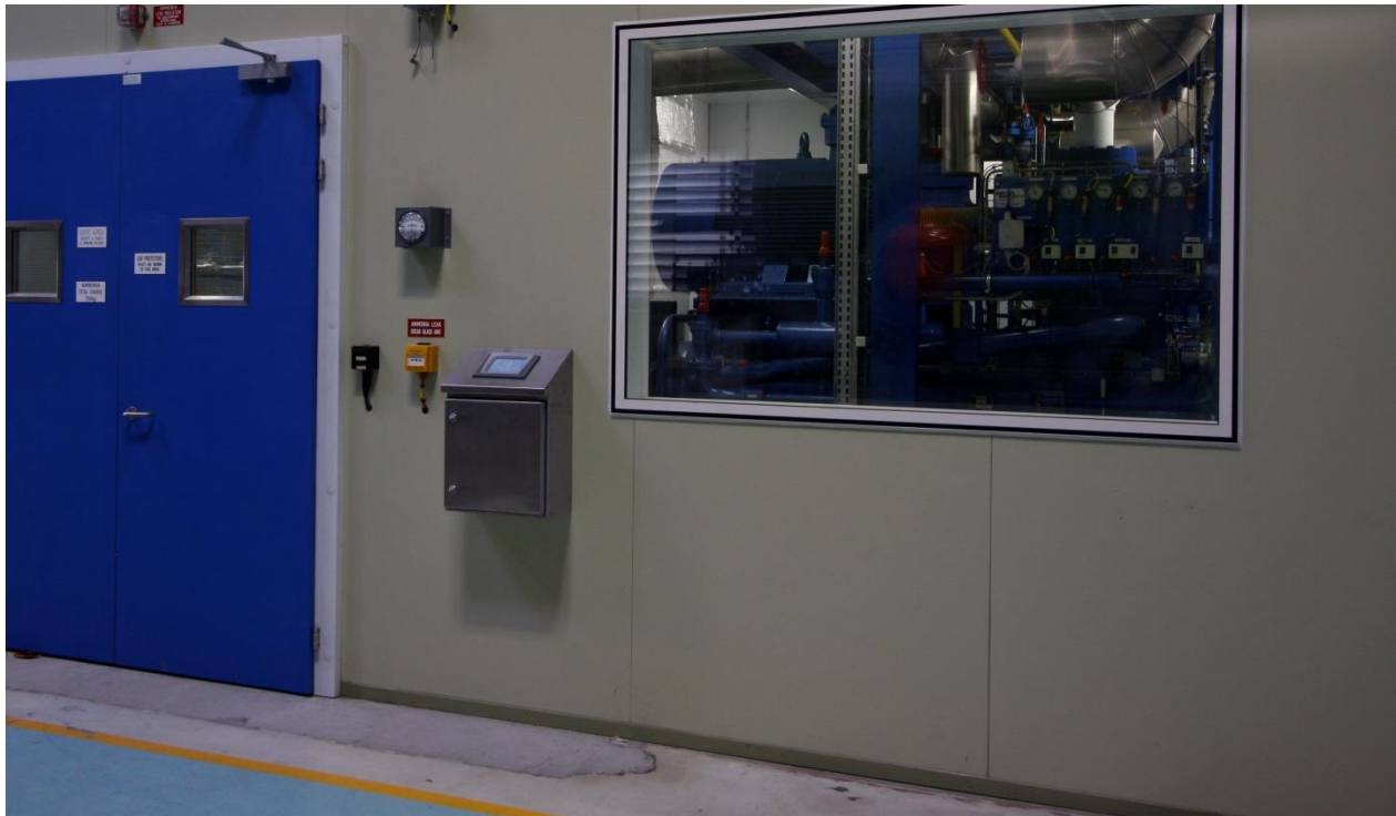
BECAUSE OF HIGH NOISE LEVELS INSIDE THE ROOM, THEY INSTALLED ONE VISION570™ OUTSIDE CONNECTED VIA CANBUS TO THE VISION280™ UNITS.
