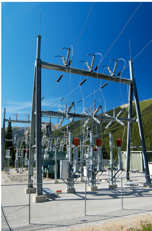
Figure 2: Much of the data needed to effectively monitor and control a power distribution system is found at substations, but collecting these data can be challenging.
