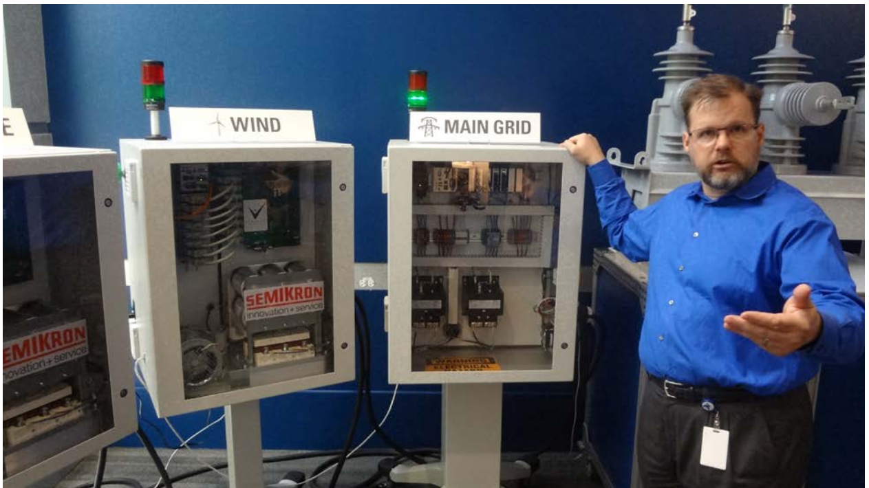
1. National Instruments uses time-sensitive networking to manage its power microgrid.
