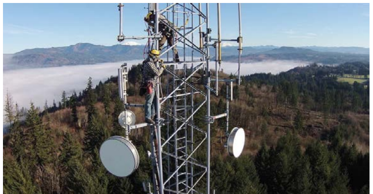
1. Wireless communications systems are clearly visible by their tower-mounted antennas pointed in the direction of a wireless link's other terminal. (Courtesy of Stephouse Networks)
