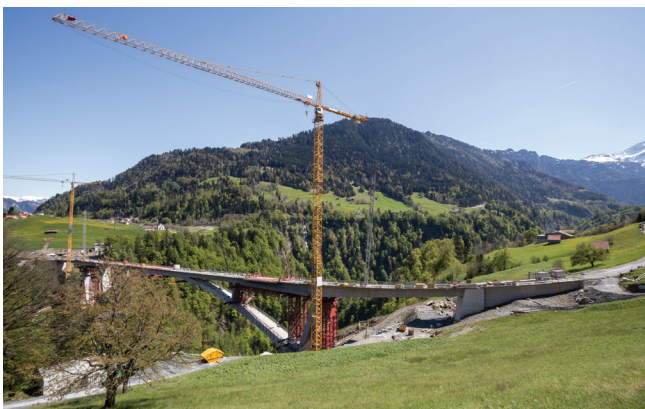
The Tamina Bridge project, built high in the Swiss Alps, presented unique design requirements. A detailed model, developed in Allplan software, proved the viability of the slender cross sections and helped secure the winning bid.
