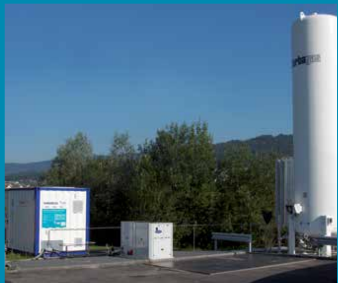
Wedeco ozone plant at the Wueri wastewater treatment plant in Regensdorf, Switzerland.
