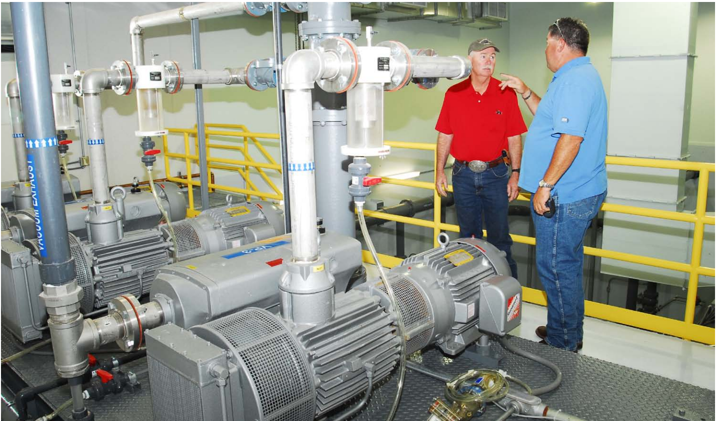
Sewer System Manager Dennis Steele (right) discusses operating details with Technician Tym Fowers inside one of Hooper's new vacuum stations.
